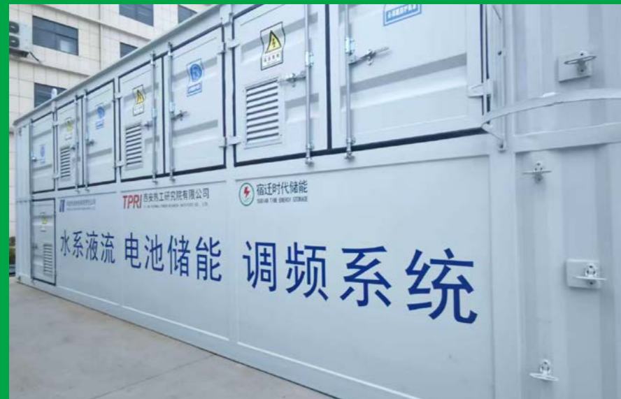
500 kW / 1,000 kWh aqueous organic flow battery system for frequency regulation, Phase II project in Luoyuan, Fujian, 2026
