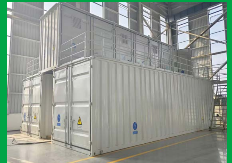
150 kW / 600 kWh iron-chromium flow battery system for long-duration energy storage (South Africa in 2026)
